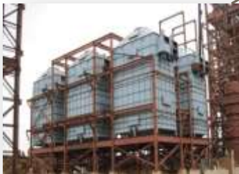
COAL GASIFICATION PLANT FOR JINDAL STEEL
