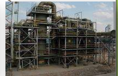
GAS CLEANING PLANT FOR KCM, ZAMBIA
